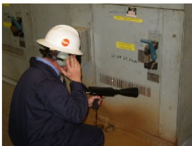
SCANNING 4160V SWITCHGEAR
