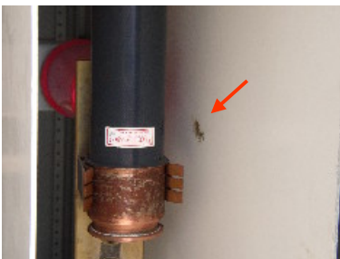
TRAKING ON 13KV SWITCHGEAR
